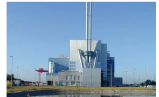
Biomass power plant Dürenrohr, equipped with REITZ fans. Photo: AE&E Inova, Köln
